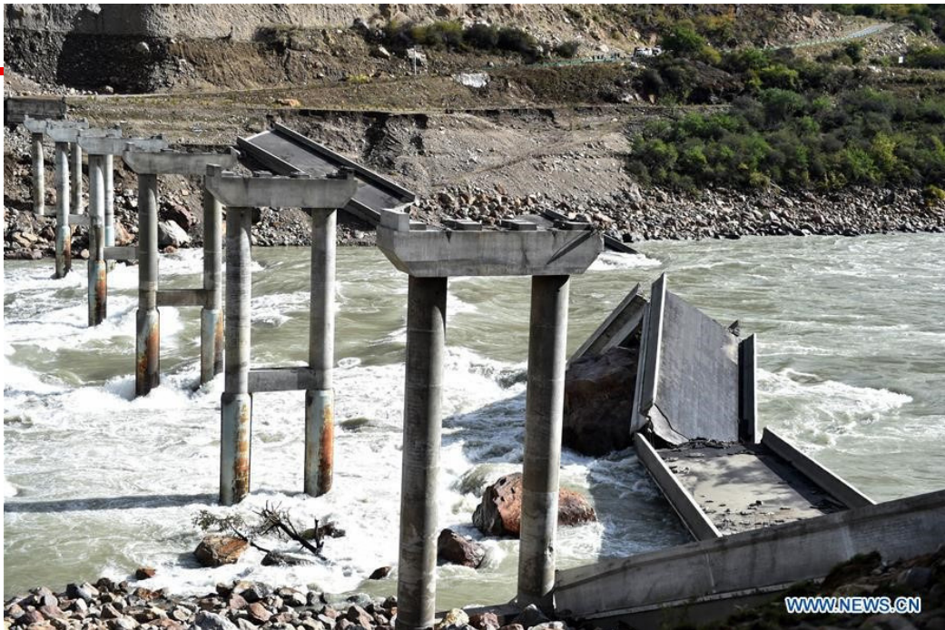
Dalin bridge, damaged by rushing water from a landslide-caused barrier lake on the Yarlung Tsangpo River in Menling County (Xinhua/Chogo)
